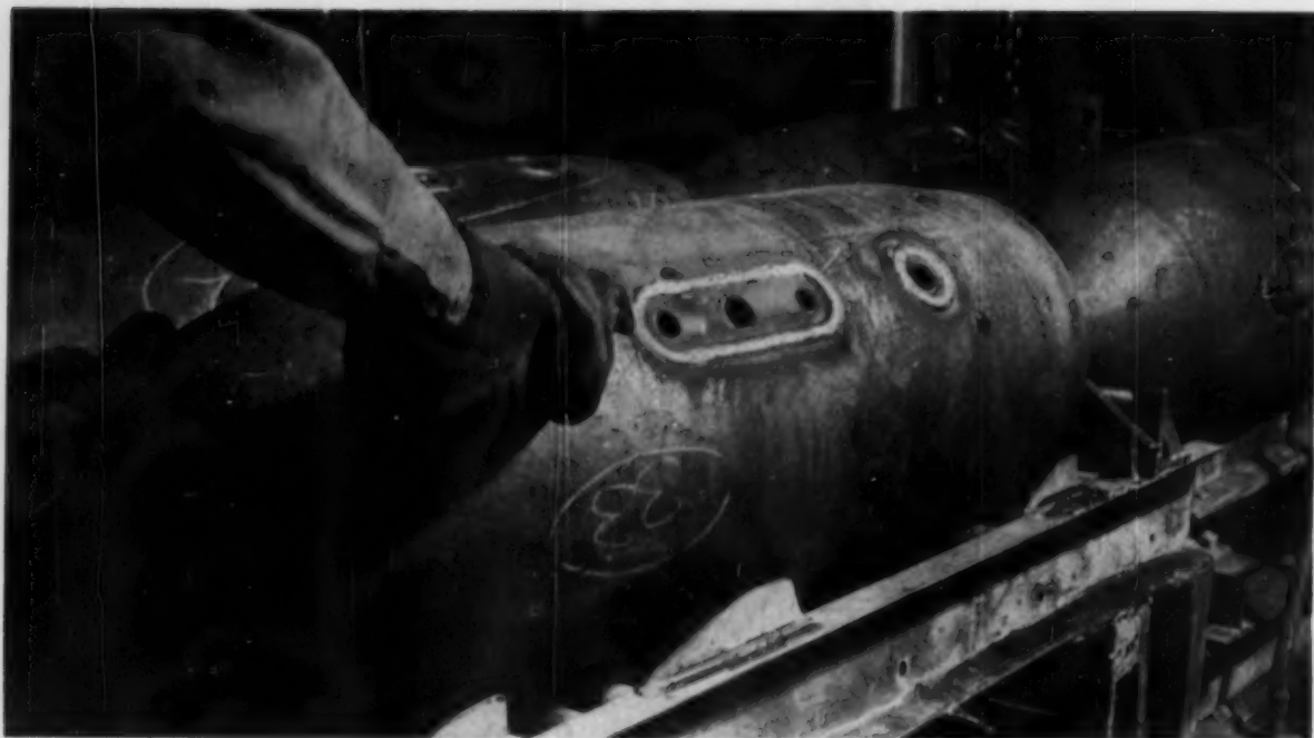
Finished welds made by the four-at-a-time welder. Inserts are forgings to accommodate materials handling equipment
